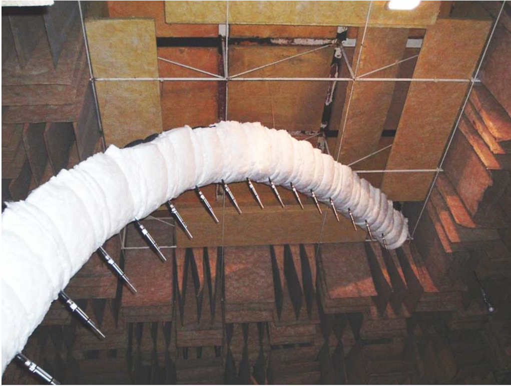
Photo 1 – Upper section of finished microphone array
